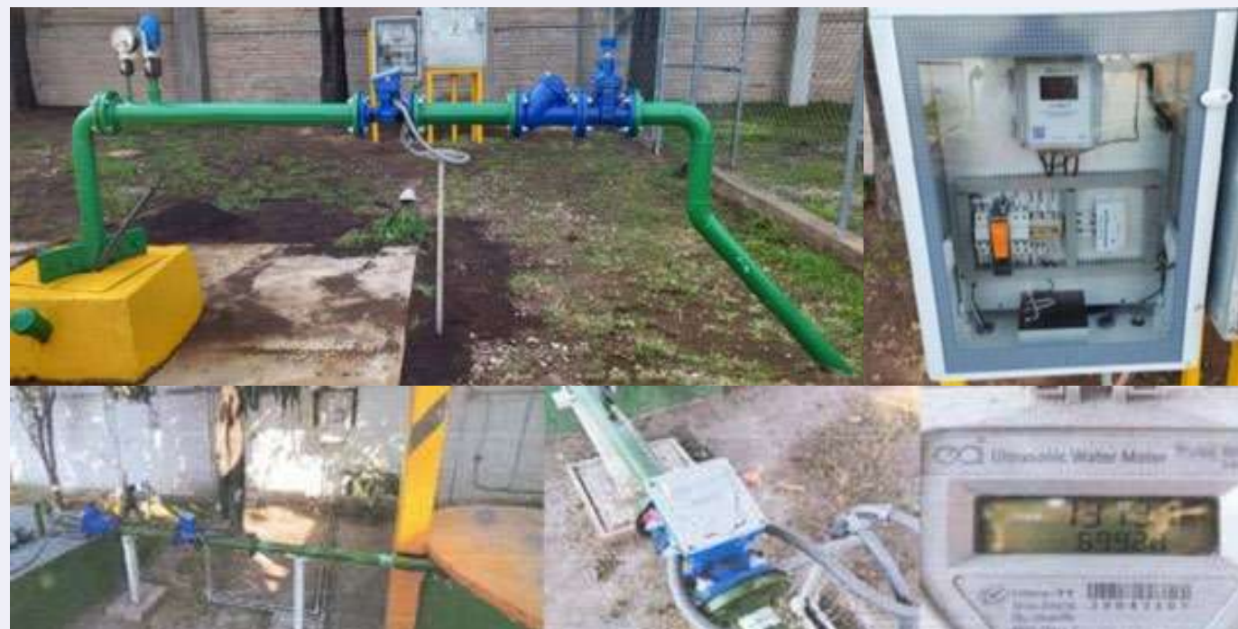
Flow meter with flow measurement system and telemetry transmission Aguascalientes Plant.
